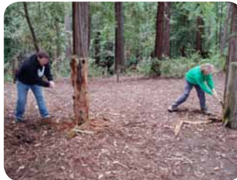
The decrepit Apache gateway being torn down and subsequently replaced during the work party.
