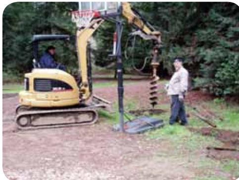
New post holes being drilled during the replacement of the rotting fence around the redwood grove.
